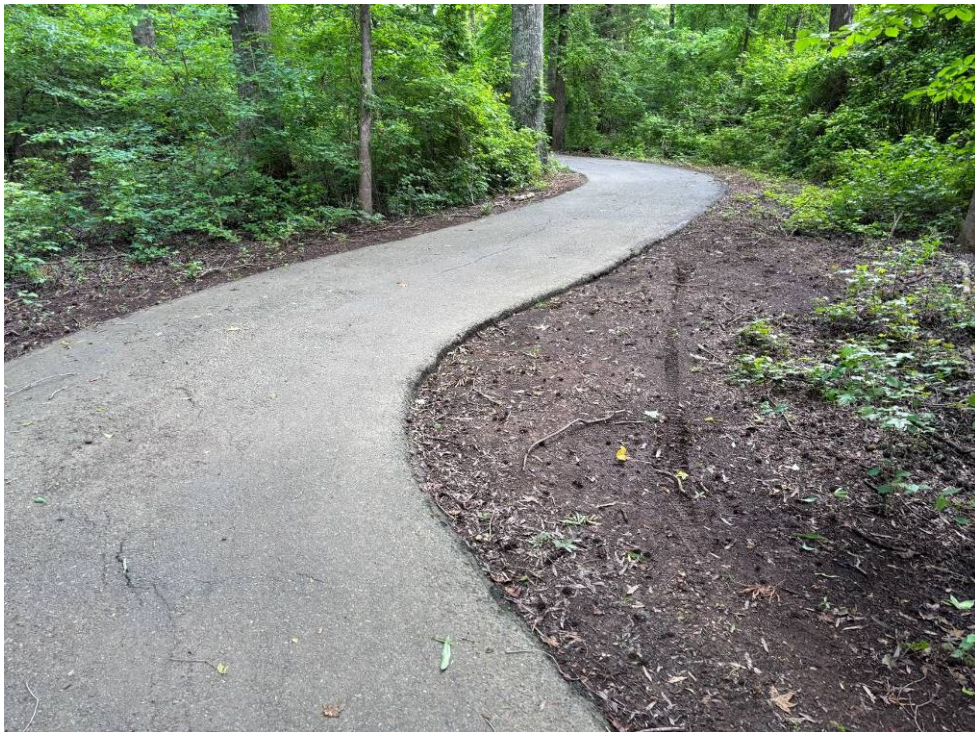
Photo 10: Northbound trail with areas of sediment build up and wet soil.
