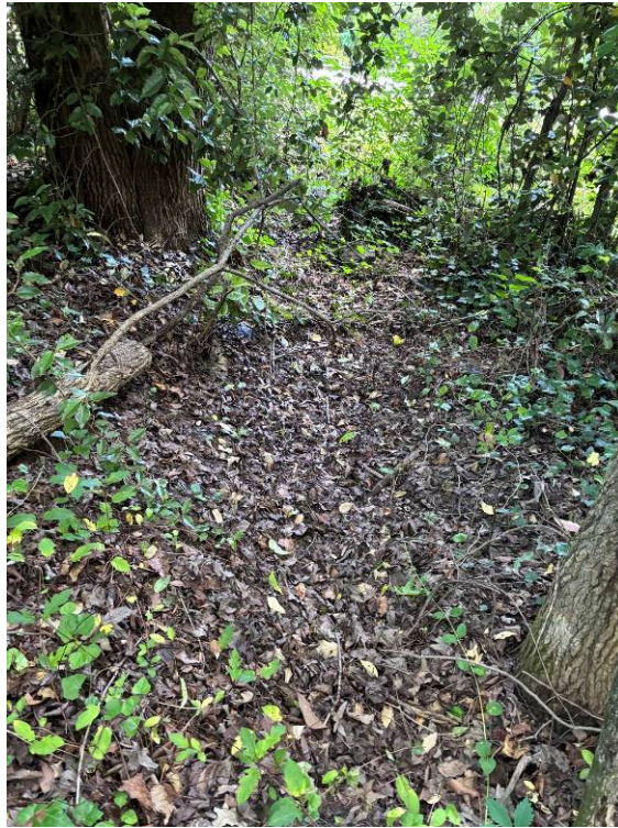
Photo 13: Accumulation of debris and sediment at the end of the shallow swale preventing positive flow into roadside ditch.
