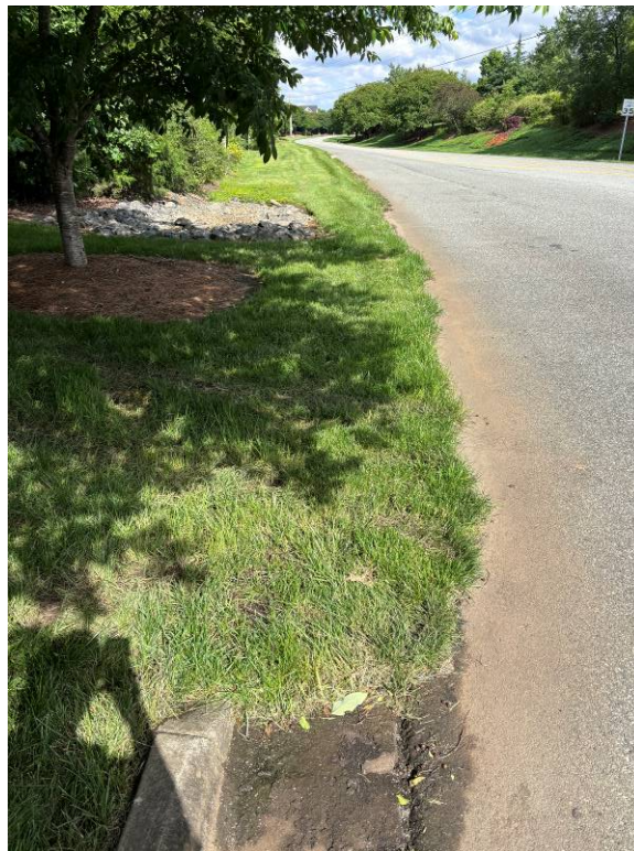
Photo 4: End of curb and riprap for storm drain outfall along Joe Kerr Road, looking west.
