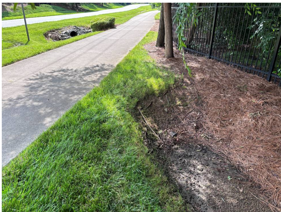
Photo 16: CMP pipe from adjacent residential area to the culverts under Joe Kerr Road. Pipe is almost completely buried.
