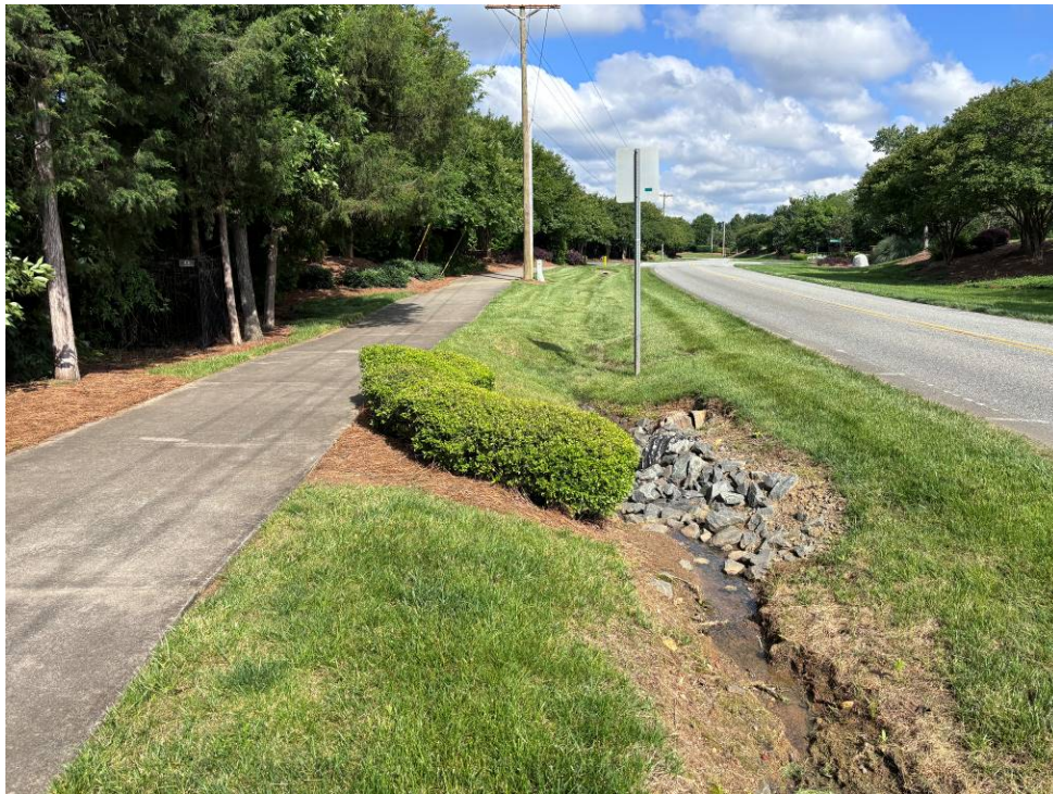
Photo 13: Confluence of the roadside ditches, culverts under the trail and road culverts.
