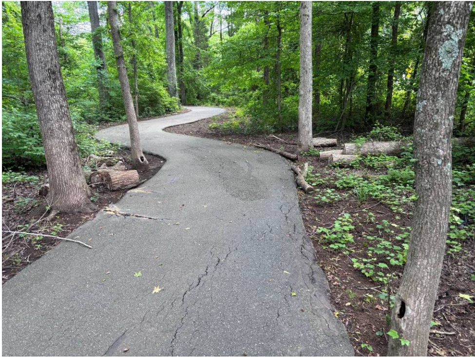
Photo 9: Northbound trail with areas of sediment build up and wet soil.
