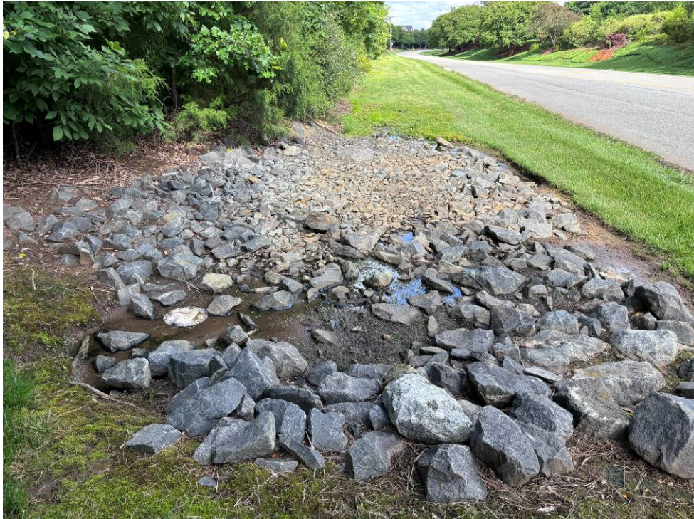
Photo 5: Riprap at outfall of storm drain system (inlets along Autumn Blossom Lane) Outfall pipe is partially buried.
