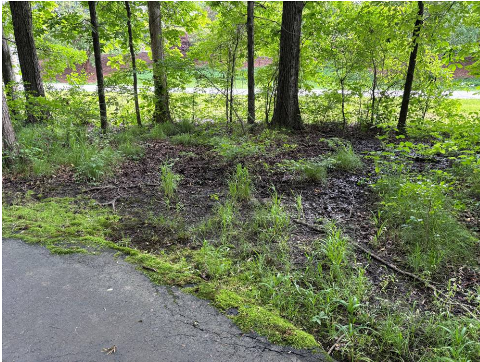
Photo 9: Trail heading west. Sediment and wet soils between the trail and road.
