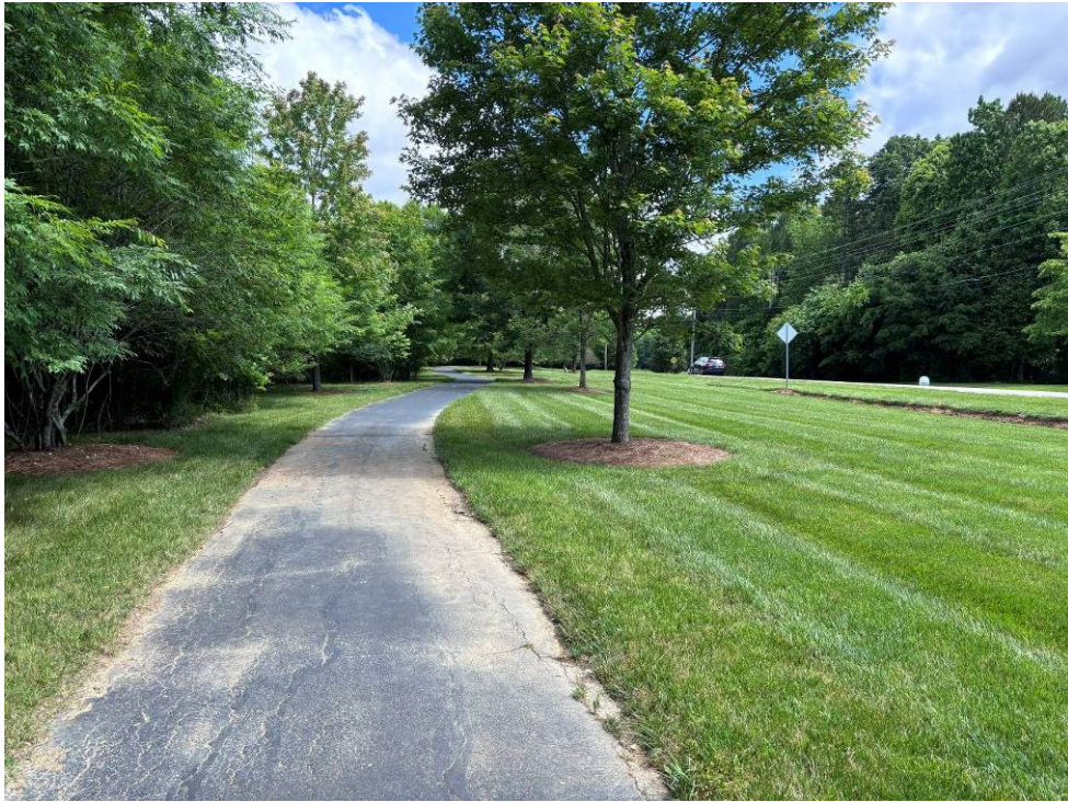
Photo 15: Northbound trail. Note discoloration on the trail where water ponds.
