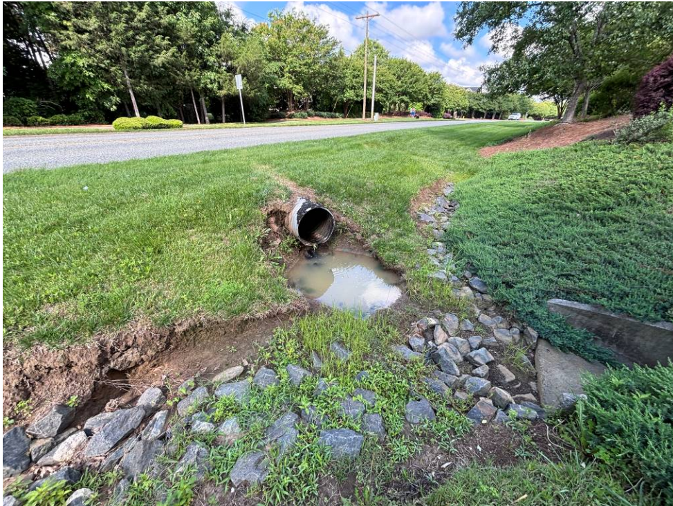
Photo 21: Downstream end of the CMP culvert under Joe Kerr Road. Outfall of the RCP culvert is in the background.
