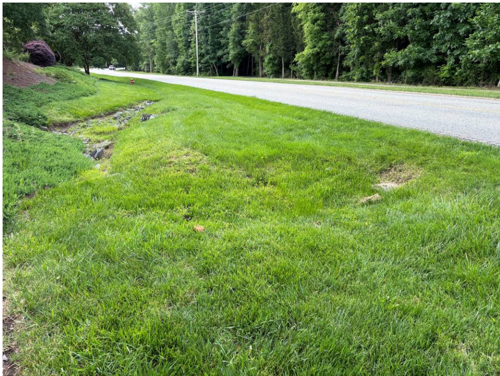
Photo 22: Outfall of the RCP under Joe Kerr Road. Outfall of the CMP culvert is in the background.
