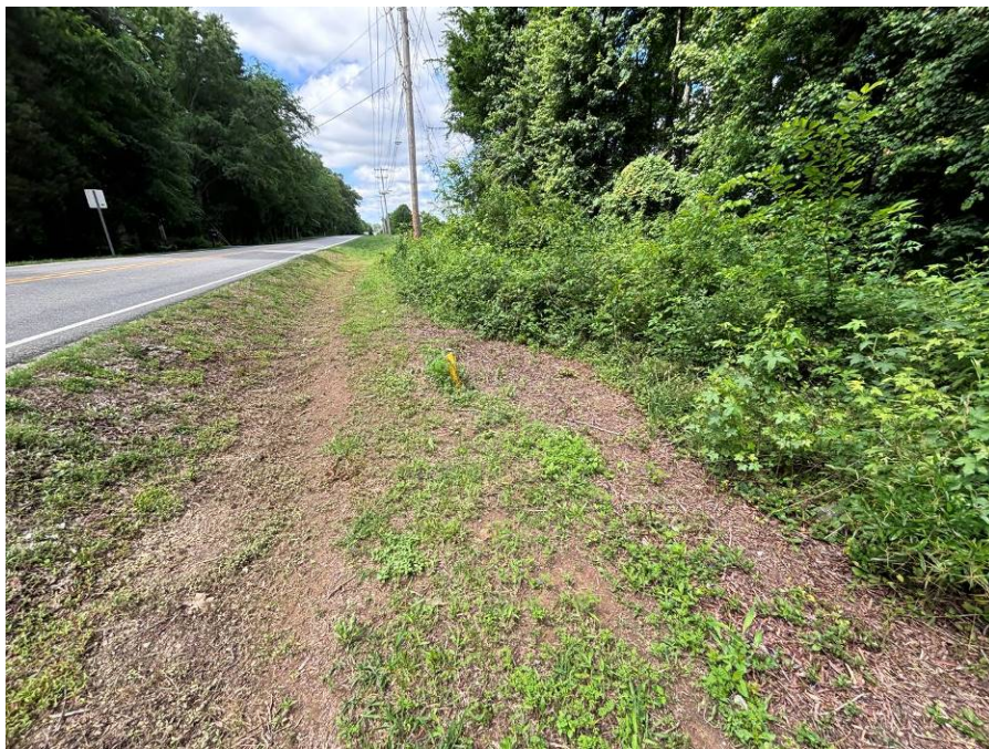
Photo 22: Existing ditch along wood line, note debris accumulation along the brush indicating runoff flowing into the woods. Culvert under the road is near the utility pole in the background.
