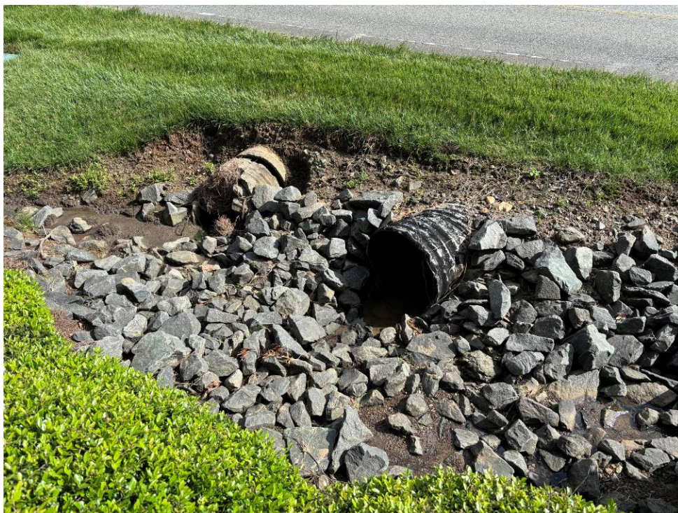
Photo 14: Upstream end of the culverts under Joe Kerr Road. Note the RCP on the left is broken and clogged.
